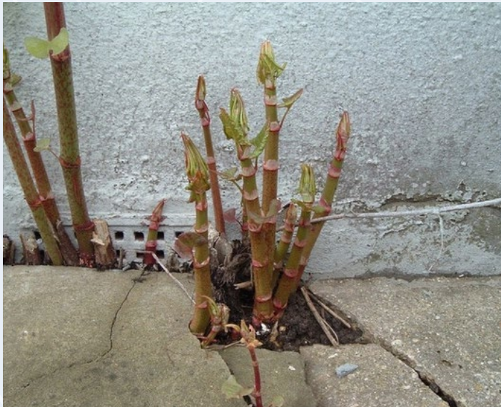
Young knotweed stems growing along a building foundation, showing how the plant can exploit cracks and cause structural damage. Photo: Sumas First Nation
