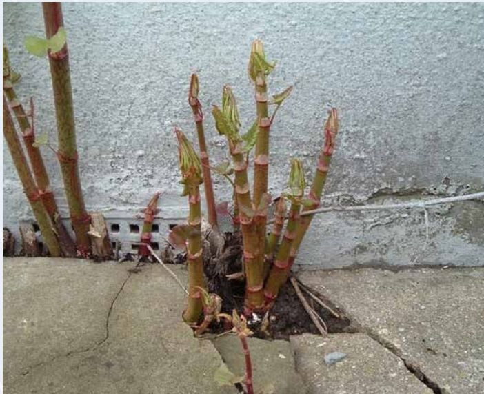
Young knotweed stems growing along a building foundation, showing how the plant can exploit cracks and cause structural damage. Photo: Sumas First Nation
