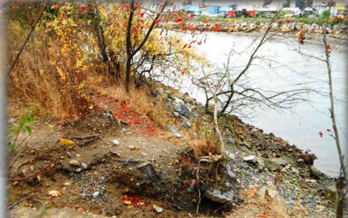
Beaver Damage & Bank Erosion
