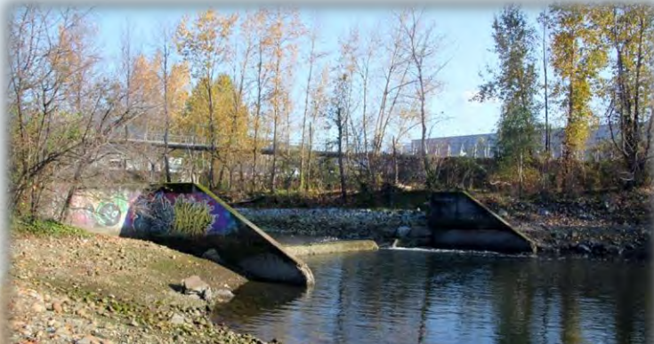
Weir Blocked Fish Passage
